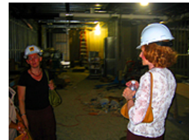
Angeliq Feuillet from Planning, Design and Construction, and Associate Dean McGovern inspect the moot courtroom's progress.
