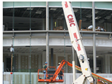
Interior walls and ceilings are completed as the exterior glass begins to enclose bay window.
