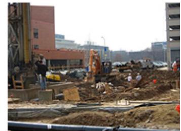
3.13.06: Excavating additional ground for foundation. Major drainage pipe and connecting line laid in soil.
