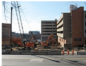
2.14.06: After groundbreaking: Heavy equipment clears the land while drilling begins for caissons for the foundation.
